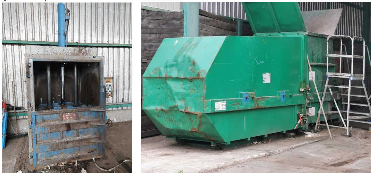
Figure 9: Compactor and Press Container
