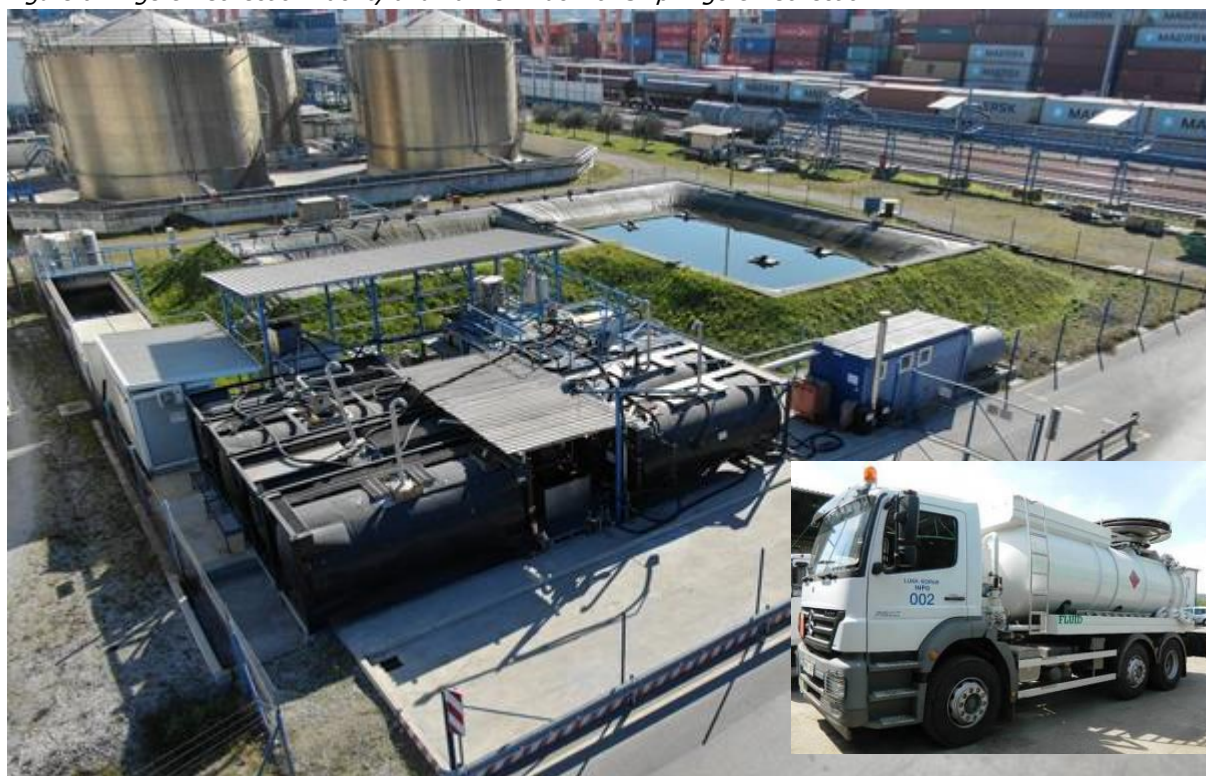
Figure 6: Bilge Oil Collection Facility and Tanker Truck for Ship Bilge Oil Collection
